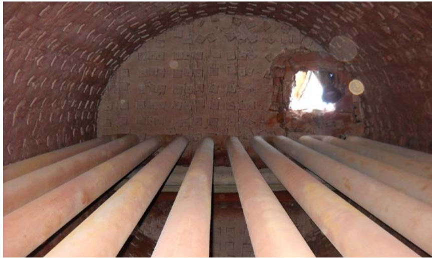
Figure 14 – Inside the Radiant Section of Heater H-31
