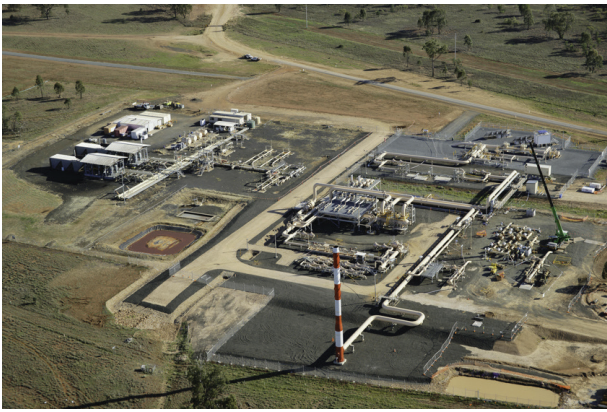
Figure 1. Using the Well Manager, technicians can manage the turn-up, turn-down or rapid shut-in of wells across a hub, by priority group, from a remote location.
