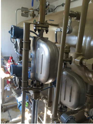
Micro Motion F-Series meters installed in well site gas allocation
