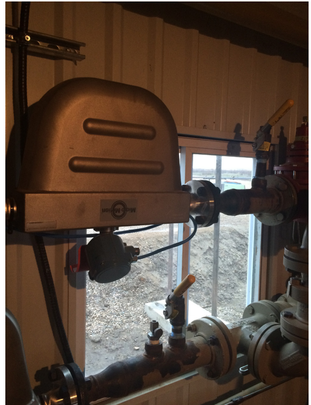
F200 meters in wet gas application for both high and low pressure lines off a heater-treater
