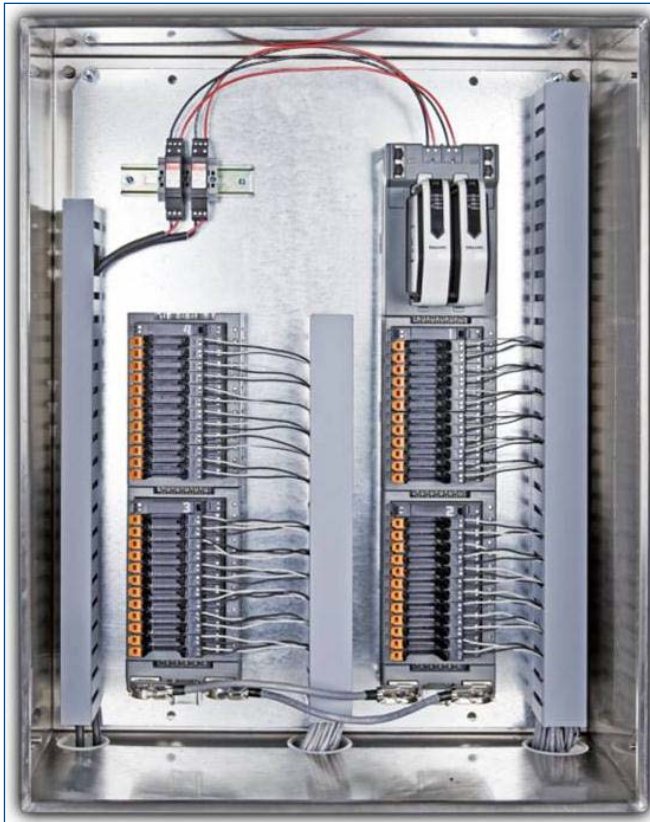
Figure 4 — Electronic Marshalling Field Junction Box with 48 CHARMs.
