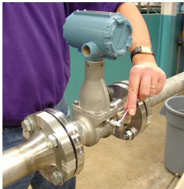
An installed Rosemount 8800 Vortex flowmeter combined with the CriticalProcess™ Vortex (CPA).
