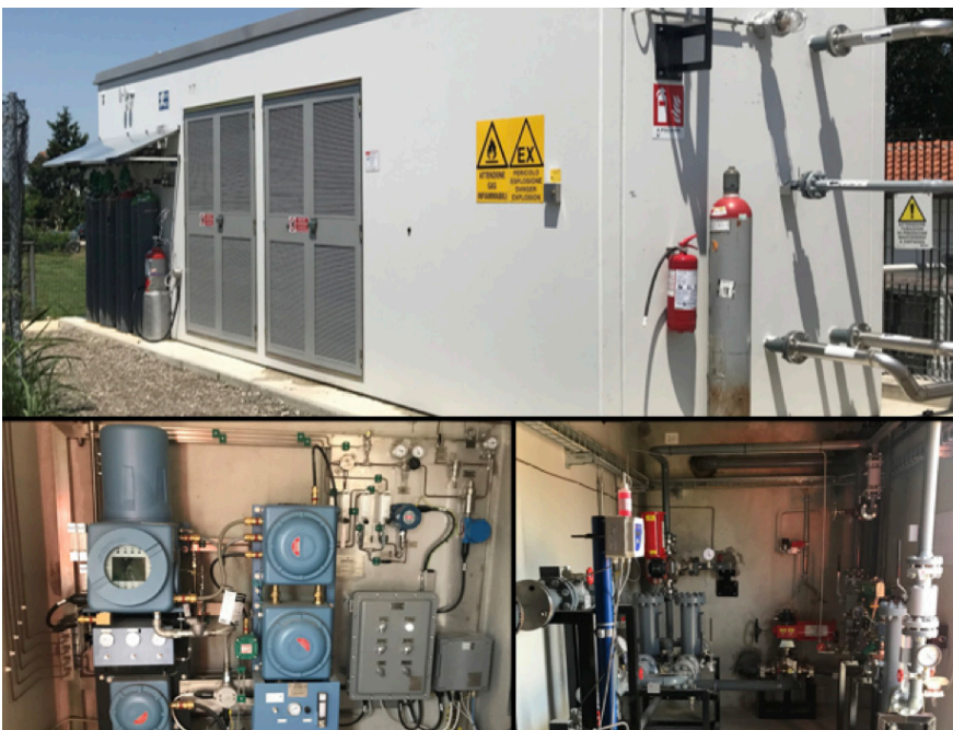
Figure 5: A biomethane injection skid can receive renewable natural gas from a processing area, analyze it to confirm it meets specification, odorize it and meter the gas for custody transfer and injection.
