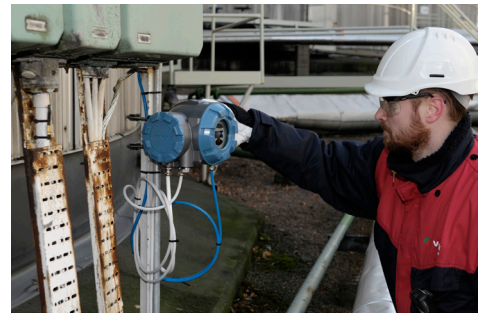
The Rosemount 2410 Tank Hub mounted at the bottom of the tank where power is already available and the display is easily accessed.
