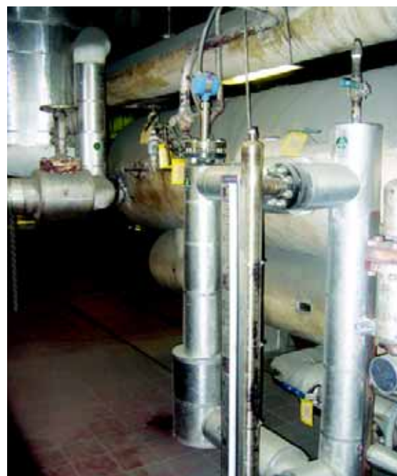
The Rosemount 3301 Guided Wave Radar Installed at the Sunbury Generation power plant.
