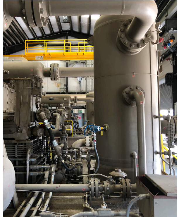
Rosemount 2140:SIS Vibrating Fork Level Detector installation
