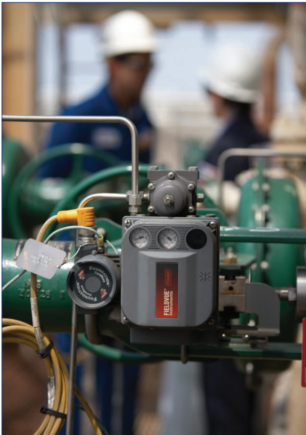
Figure 3. Intelligent digital valve controllers identify maintenance problems before they affect operations.
