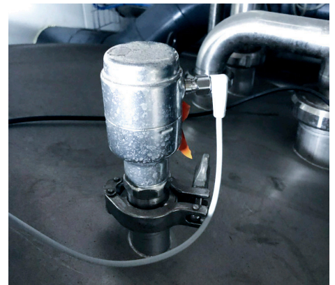
Image 1. The Rosemount 1408H is installed on the brine tank.
