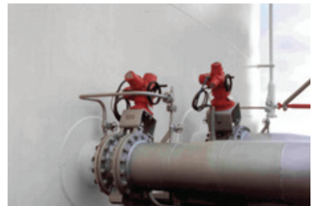
FIG. 1 - Example of TOVs installed in tank farm applications for liquid hydrocarbon services
