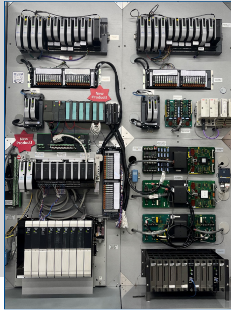
Solutions for ABB Bailey and Siemens Systems.
