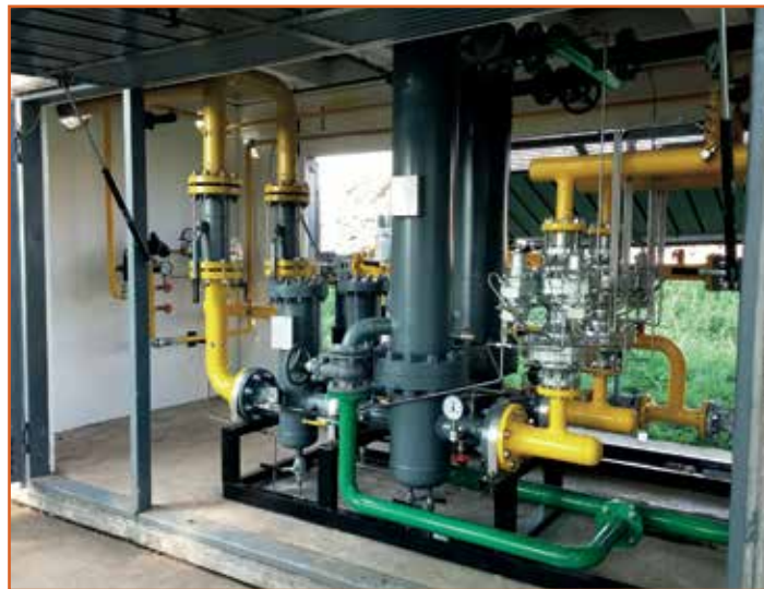
Pressure reducing and metering station
