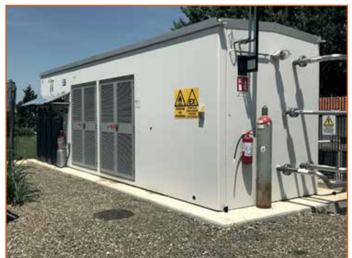
Biomethane injection skid – building
