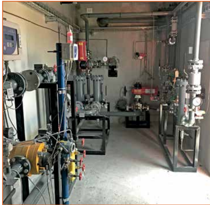
Biomethane injection skid – inside
