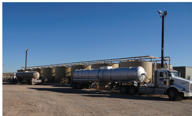
FIGURE 2. The loading facility handles up to three trucks at the same time. (Source: Emerson Process Management)
