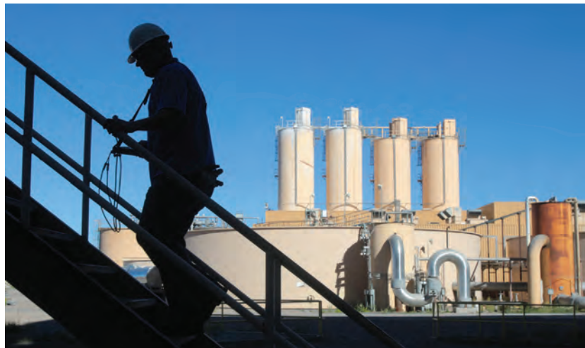
Figure 2: TEP employee Gary Gardner, who is part of the predictive maintenance group, walks throughout the generating station in Springerville, collecting data where he measures ultrasonic, vibration analysis, infrared thermography and electrical motor testing, analyzing equipment to predict when it will need replacing.
