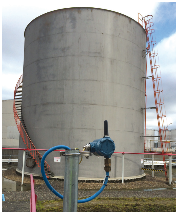
Figure 3: Tank farms cover large areas that are remote from a refinery's control system, but near enough for wireless transmitters to reach the control system.
