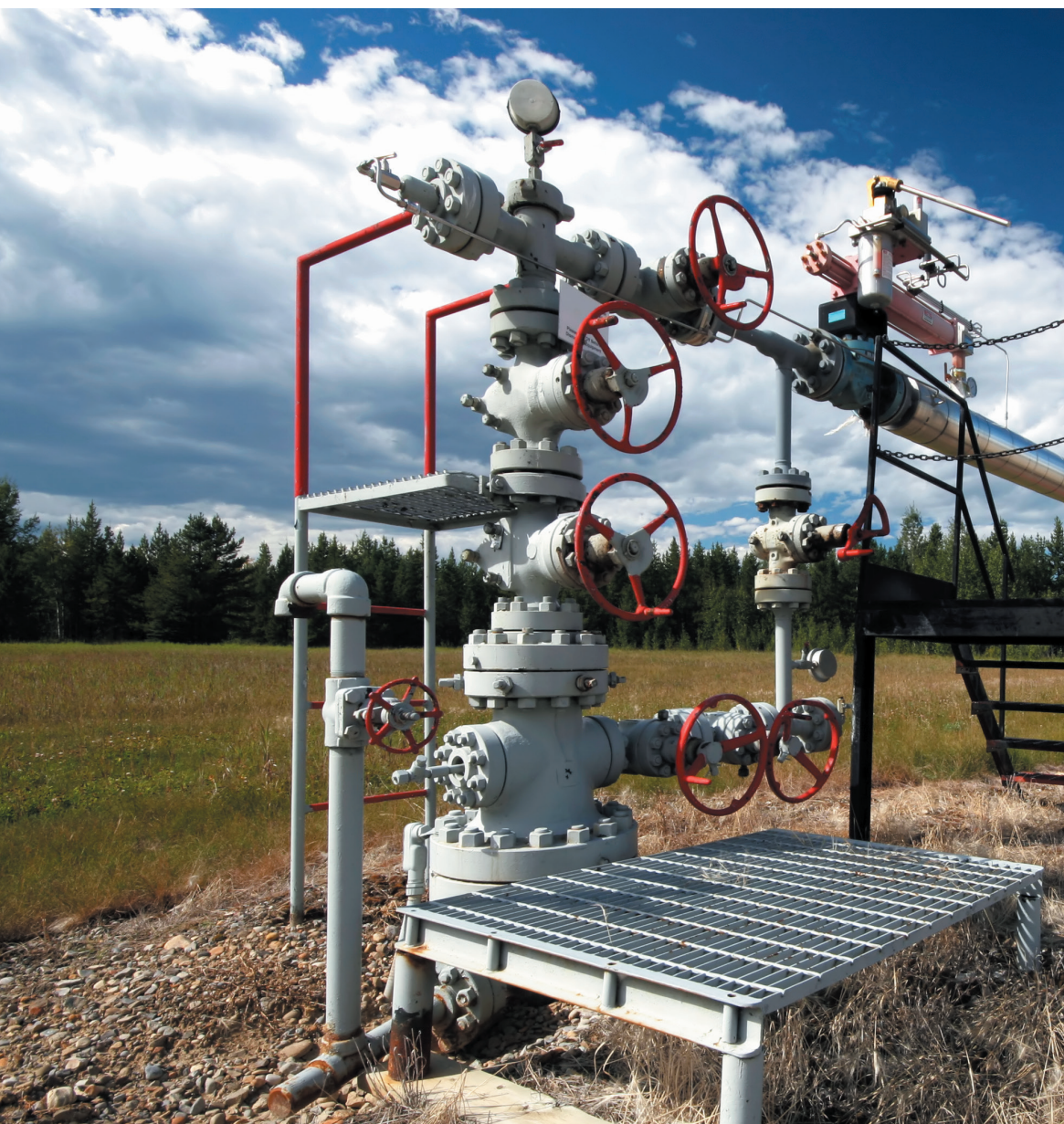
Figure 4: One oil producer added more than 3,500 WirelessHART devices to wellheads without needing additional power at the sites.
