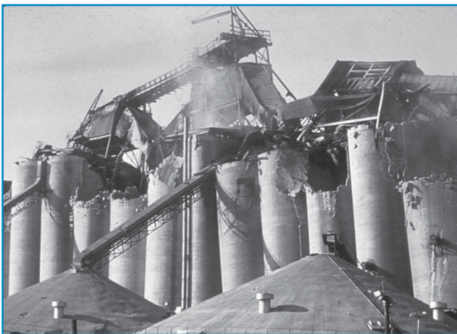
ELIMINATING DISASTERS LIKE THIS REQUIRES CAREFUL CLASSIFICATION OF AREAS AND THE USE OF THE PROPER ELECTRICAL EQUIPMENT.
