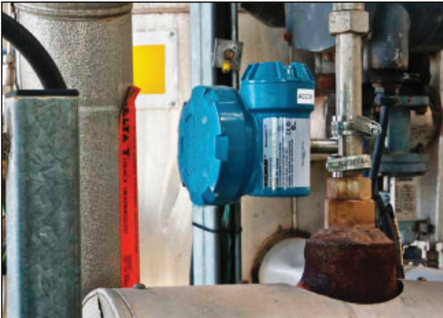
Figure 4 - Acoustic monitors mounted next to steam traps took less than ten minutes per trap, and the system paid for itself in energy savings within a year
